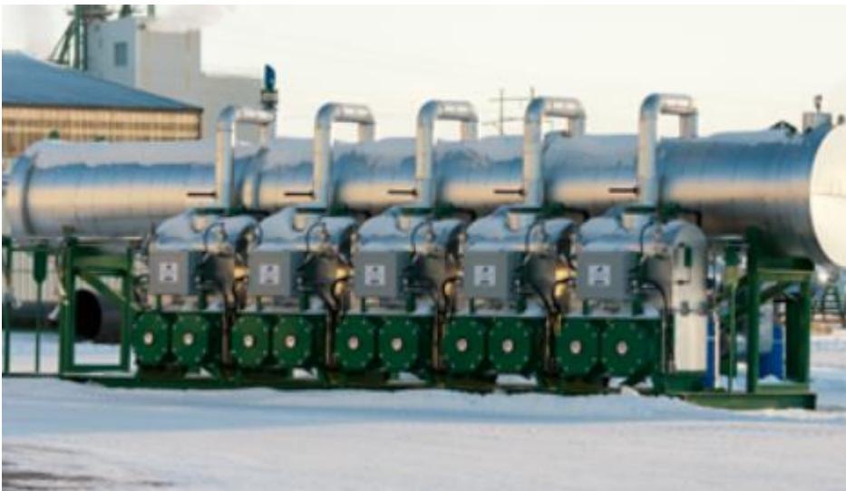
Fig. 7 3.85 mmBTU Natural Gas Line Heater
